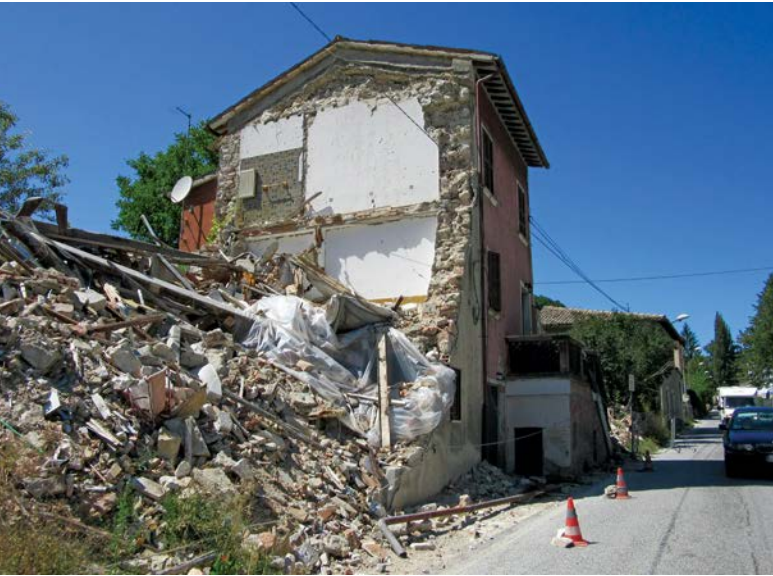
Many towns in the central Apennines were damaged during the 2016–2017 seismic sequence that hit the region. Here, rubble from a toppled building remains along a roadside in the town of Visso.
